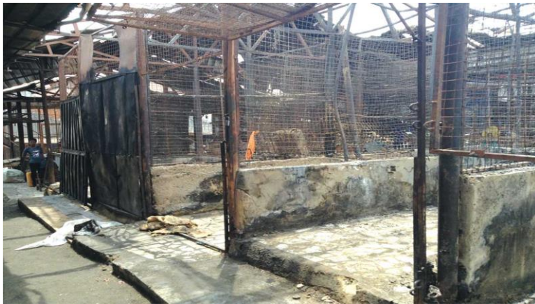
Figure 3. Burnt Shops in Garki Model market as a Result of the Use of Electricity Generator (Source: Guardian, 2016 ( https://guardian.ng/sunday-magazine/more-market-fires-than-meet-the-eye/ ); Retrieved on 06/04/2023].
