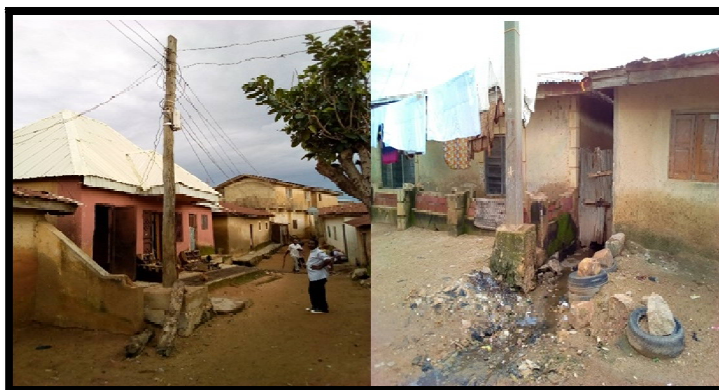
Figure 11: Location of High-Tension Power Line in Front of Houses Source: Author's Field Survey, 2018
